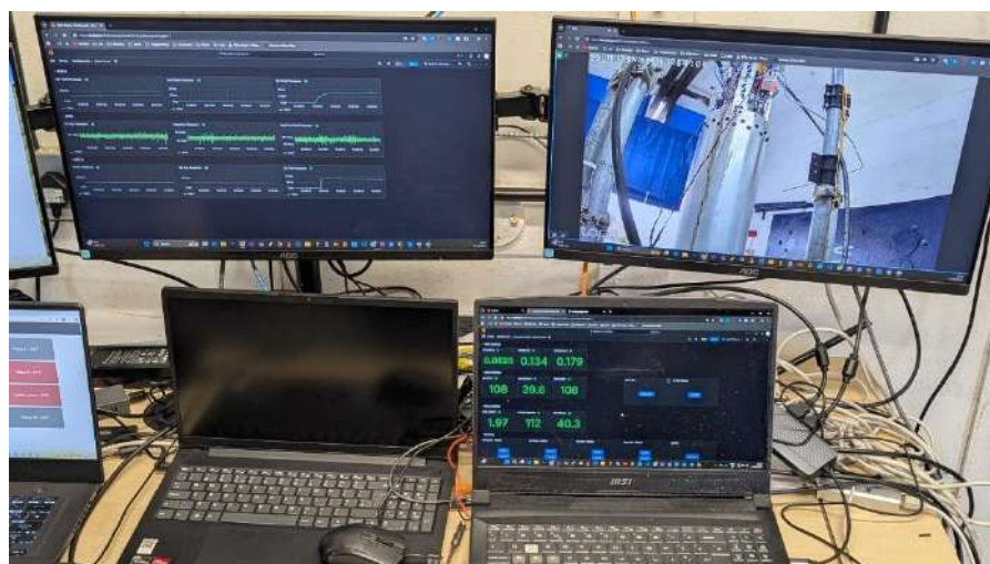
Figure 84 - A Close Up of the Control Room Displays
