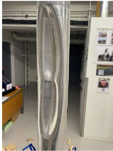
View of tank buckling
